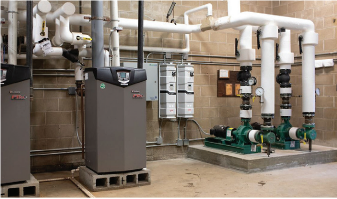
The City of Pawtucket's investment in building management systems helped to significantly reduce energy costs.
